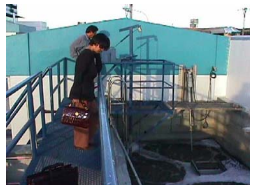
Catering Services SBR System Capacity: 60 m 3 /day
