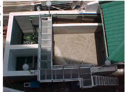
University Sewage Treatment Plant Capacity :85 m 3 /day.
