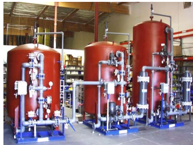
TWO BED CATION & ANION EXCHANGERS ION EXCHANGE SYSTEMS
