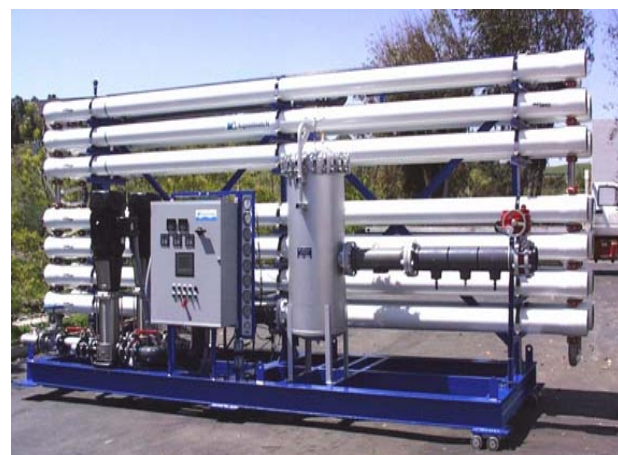
300 GPM high rejection R.O system for Nitrate Removal from City Water.
