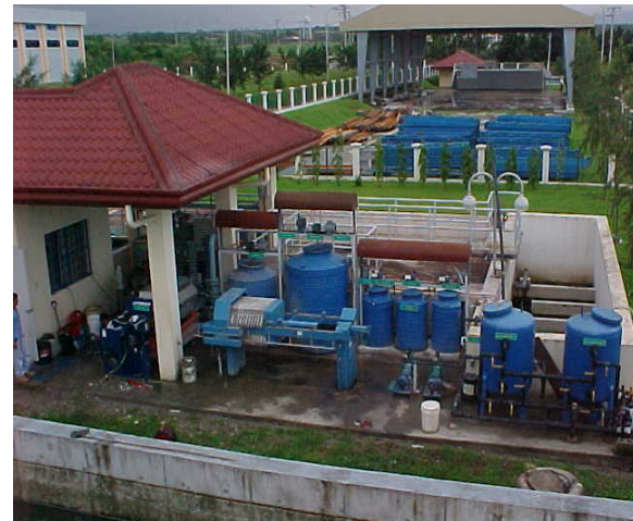
Avon Products MFG, Inc. Capacity: 60m3/day Wastewater Plant
